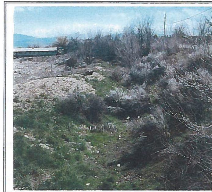
Current condition of Ditch 35, photo taken as part of the Report on the History of Water Right Lands in Agua Fria, prepared for Santa Fe County and the Office of the State Engineer, June 2005
